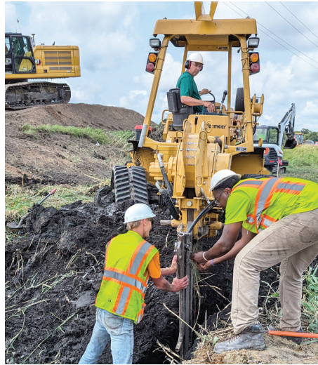
Our crew is plowing in a replacement fiber line for the one that was cut. Chris Veldhouse is in the cab while Nathan Hilbrand and Marvin Perkins guide the fiber into the plow chute.
