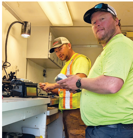
Braeden Long and Matt Lloyd repair the damage by splicing fiber optic lines in the portable trailer while on location.
